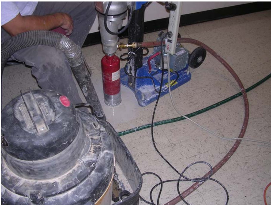
PHOTO 4 – DRILLING AT BORING LOCATION B-6 WITHIN THE HALLWAY OF THE EAST WING OF BUILDING 1.
