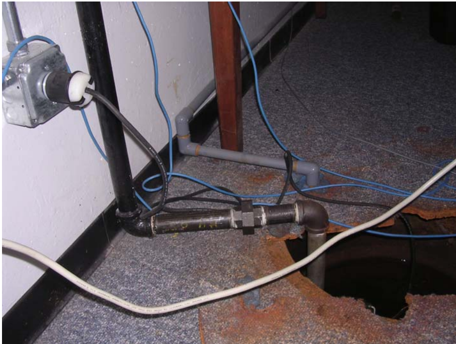
PHOTO 2 – VIEW OF SUMP B-04B LOOKING WEST, LOCATED WITHIN THE BASEMENT OF BUILDING 1, EAST WING.
