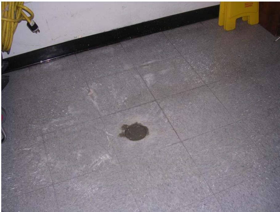
PHOTO 6 – PATCH APPLIED TO BORING B-9, LOCATED AT THE EASTERN END OF THE BUILDING 1 EAST WING HALLWAY.
