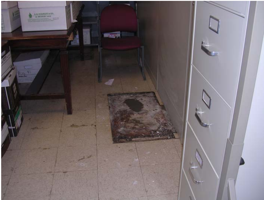
PHOTO 5 – PATCH APPLIED TO BORING B-5, LOCATED WITHIN ROOM B-16, NORTH SIDE OF THE BUILDING 1 EAST WING.
